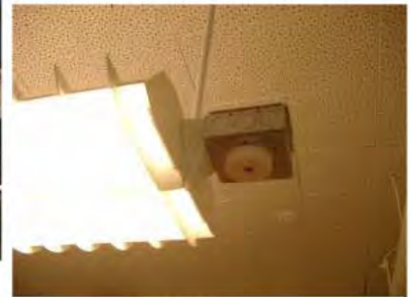
Photosensor built into luminaire
