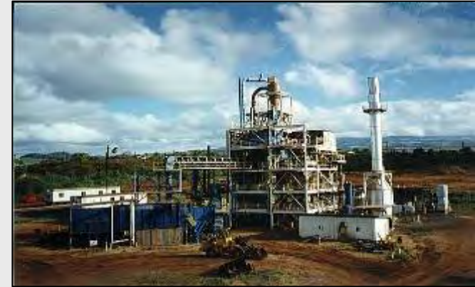
100 ton per day Bioenergy Demo Plant in Hawaii using bagasse
