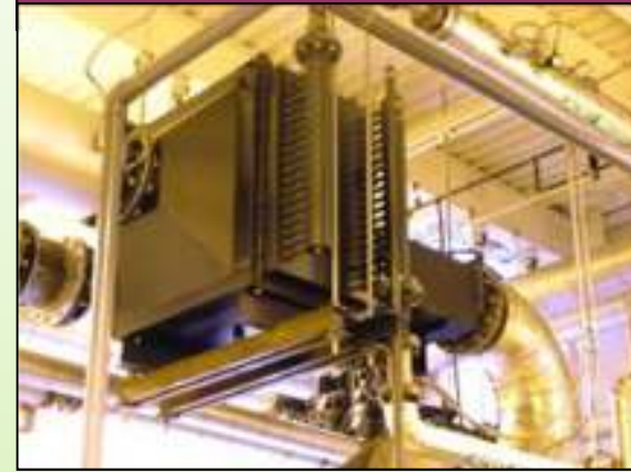
Waste Heat Recovery
