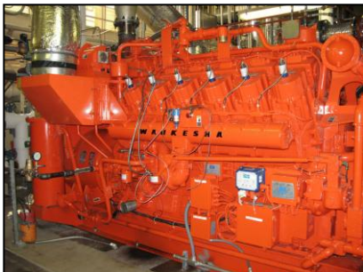
Figure 5: Waukesha 1,000 kW Lean Burn Turbo-Charged Dual Fueled Gas Engine Generator Set
