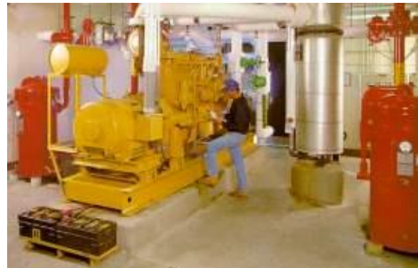
GJJWTF Existing Engine Generator System
