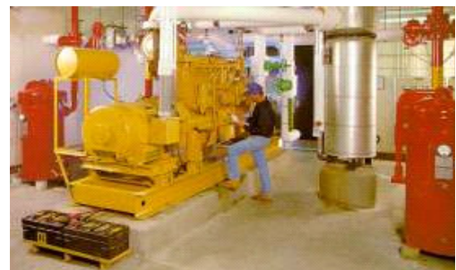
GJJWTF Existing Engine Generator System
